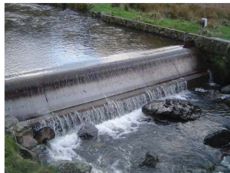
500l/s Coanda installation
